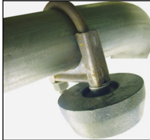
Typical mass damper
