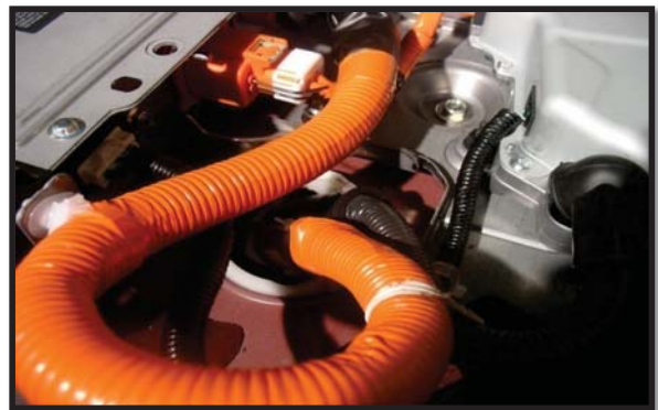
High-voltage Battery Wiring
